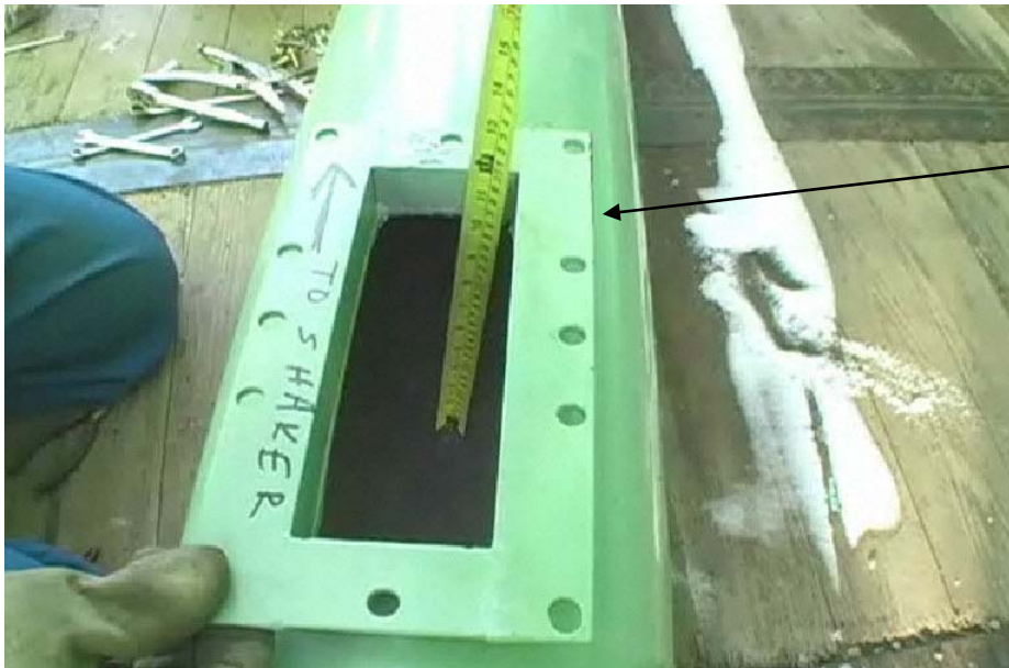
The saddle: an iron mount welded onto the flow return line
